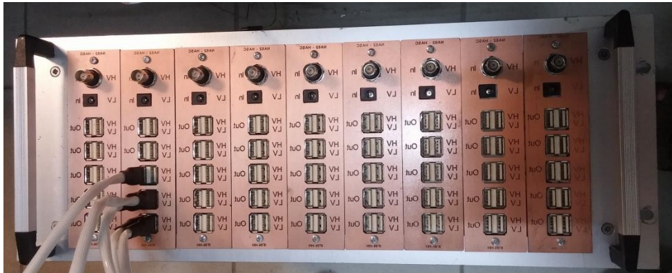
HV and LV distribution box
